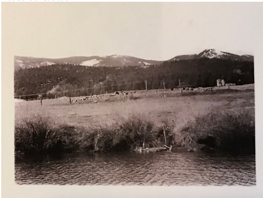
Photo HP01. House construction—foundation wall, ‘Gould Lake’ pond or North Fork of the South Platte River in foreground, buildings in background were likely located on Price’s Shawnee lots, estimated between 1940–1942, view to southwest towards Shawnee (Gould Family Photo Collection, courtesy of Nancy Kempf).
