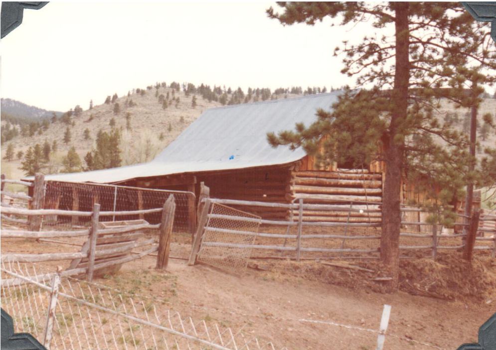
Photo HP21. West and south side of barn, with camera facing north (USFS Photo, Dargan 1979:8).
