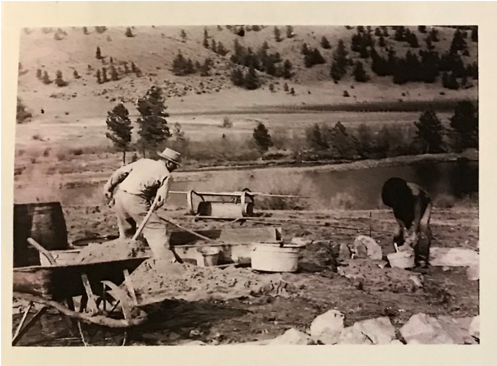
Photo HP04. House construction—pond in background, between 1940–1942, view to northeast (Gould Family Photo Collection, courtesy of Nancy Kempf).
